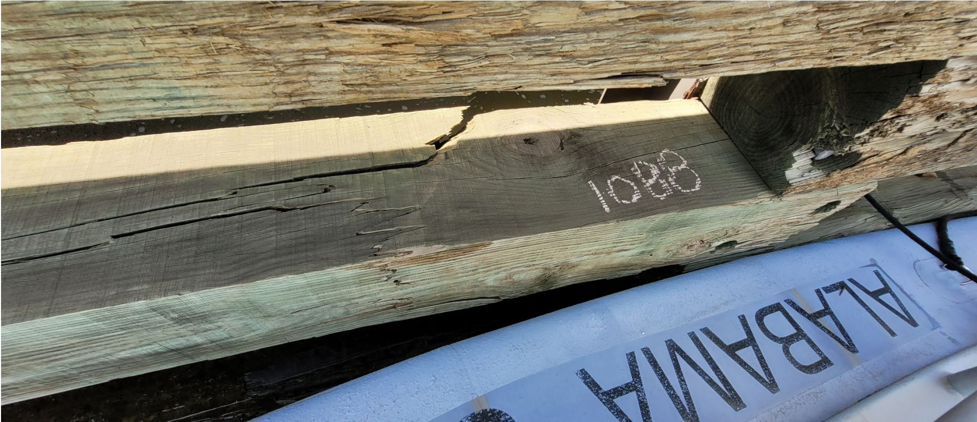
Cap Log 1087 to 1091: Replace one wooden wale, a 12" by 12" by 205" marine treated timber, and all mounting hardware.
