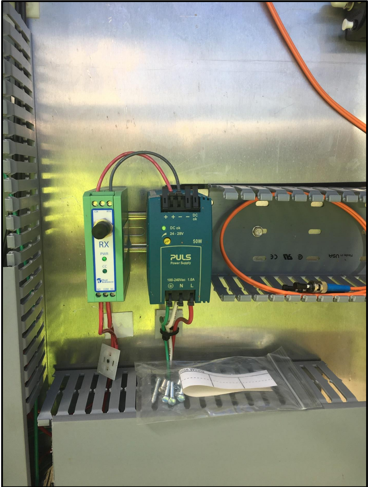
Figure 2 - Lighting Control Panel HM23-2
