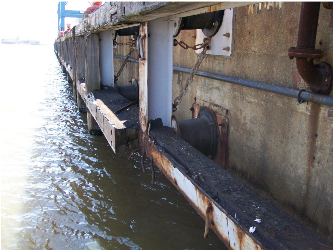
Typical Berth 2 Fender System – Looking South
