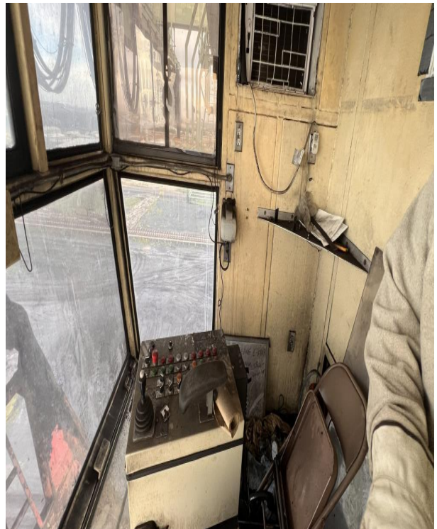
Photo 32 Comments: View of M Crane Control Cabin
