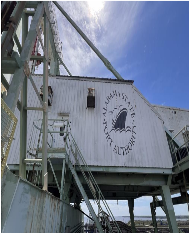
Photo 19 Comments: View of the Z Crane Mechanical Room
