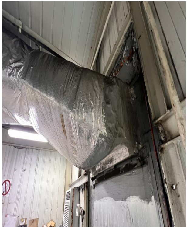
Photo 36 Comments: View of AC Duct System in Larger Mechanical Room - M Crane
