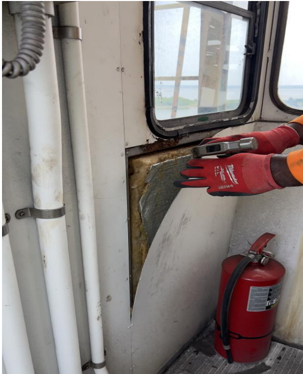
Photo 15 Comments: Suspect Asbestos Sampling - Z Crane Control Cabin
