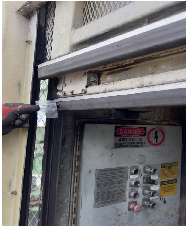
Photo 28 Comments: Suspect Asbestos Sample Collection - M Crane Elevator
