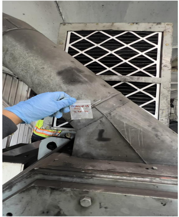
Photo 30 Comments: Suspect Asbestos Sample Collection - M Crane Smaller Mechanical Room
