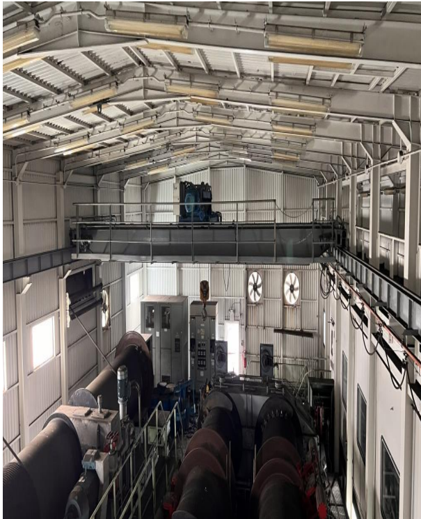
Photo 5 Comments: View of the S Crane Mechanical Room (inner)
