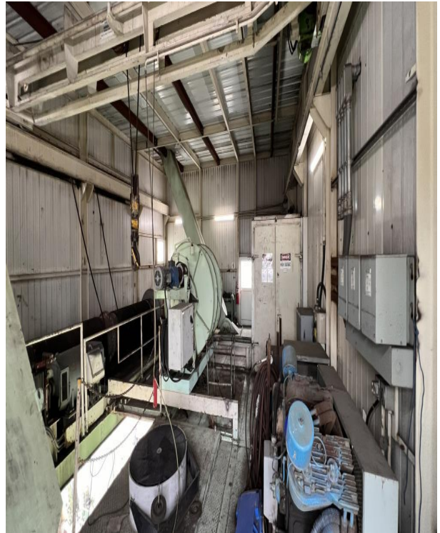
Photo 34 Comments: View of Larger Mechanical Room (inner)
