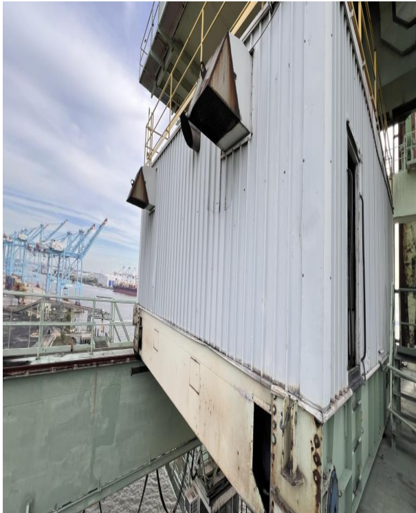
Photo 29 Comments: View of Smaller Mechanical Room - M Crane
