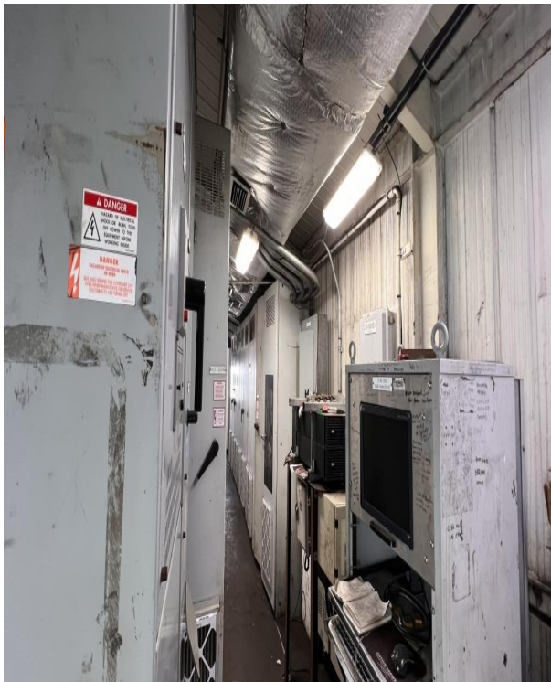
Photo 35 Comments: View of Panel Room in Larger Mechanical Room - M Crane
