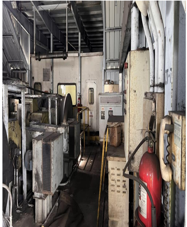
Photo 20 Comments: View of the Z Crane Mechanical Room (inner)
