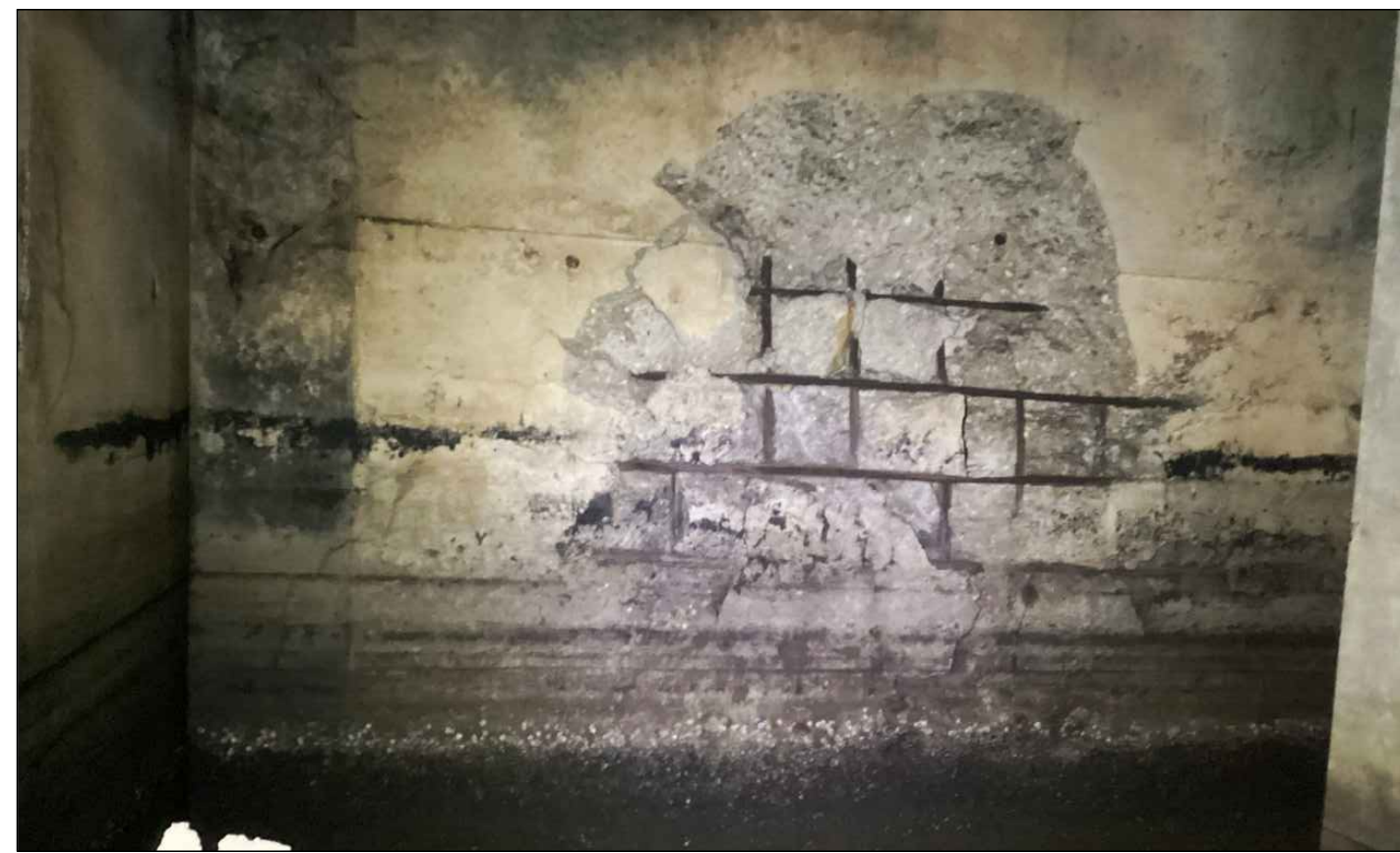
WALL DAMAGE REFERENCE PHOTO @ LOCATION 20 N.T.S.
