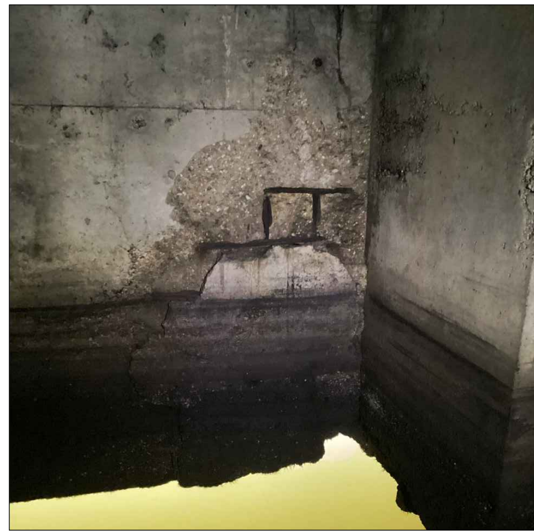
WALL DAMAGE REFERENCE PHOTO @ LOCATION 39 N.T.S.
