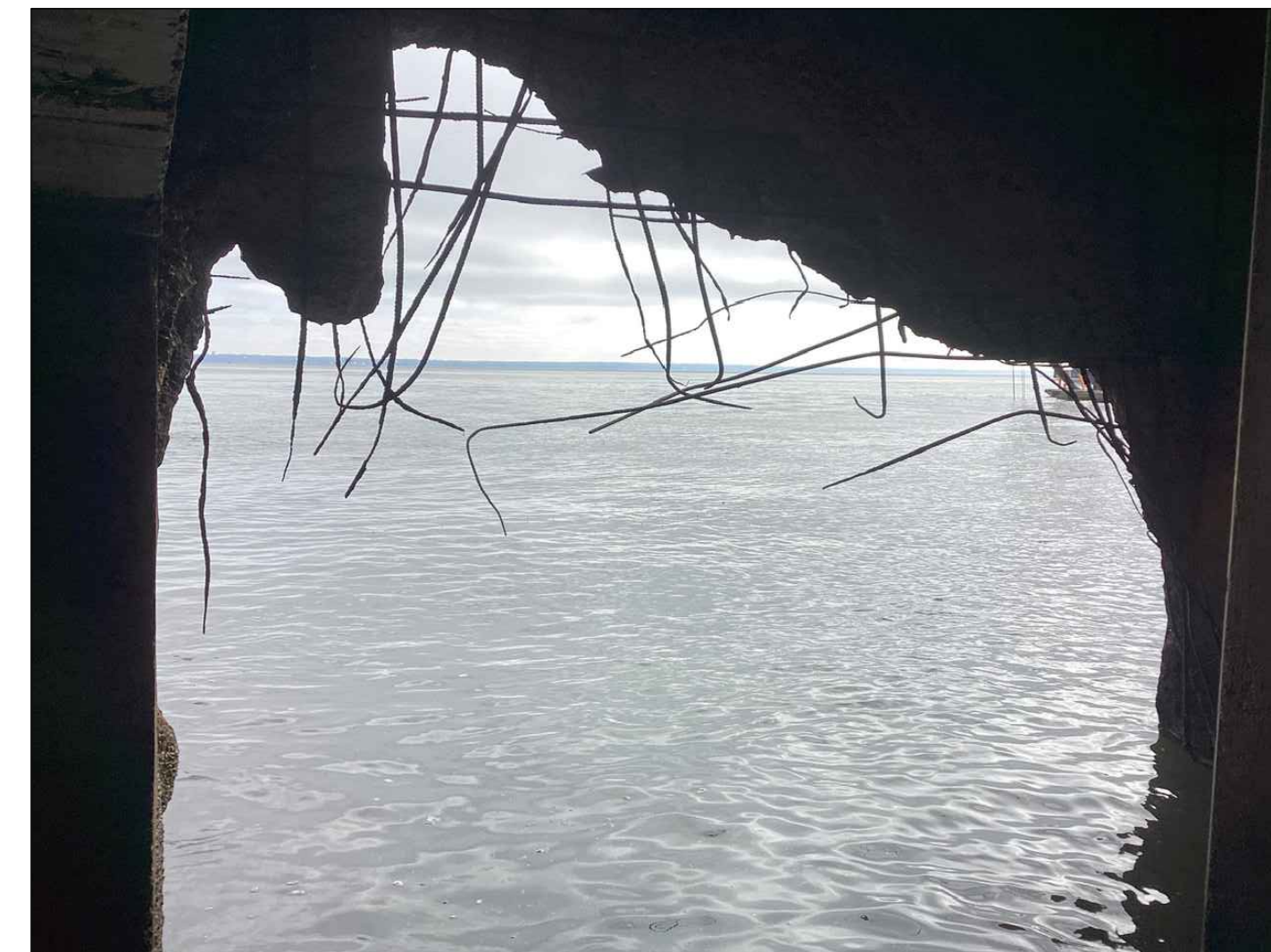
WALL DAMAGE REFERENCE PHOTO @ LOCATION 50 N.T.S.
