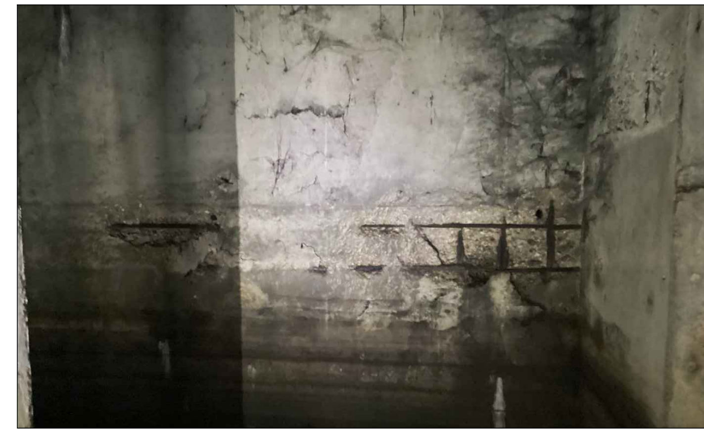
WALL DAMAGE REFERENCE PHOTO @ LOCATION 33 N.T.S.
