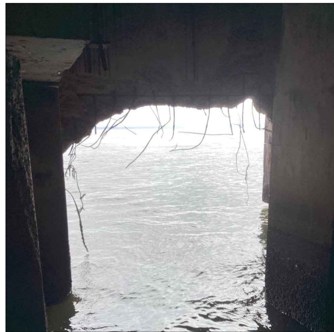
WALL DAMAGE REFERENCE PHOTO @ LOCATION 51 N.T.S.
