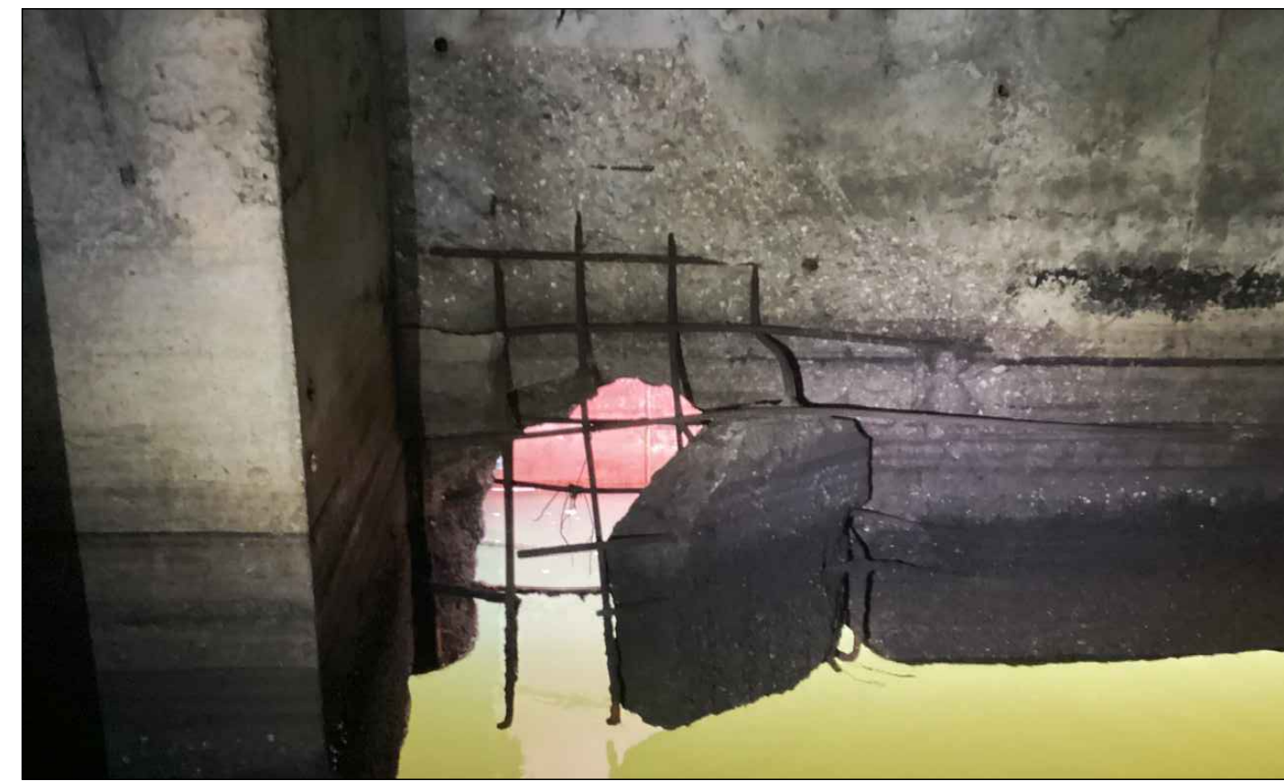
WALL DAMAGE REFERENCE PHOTO @ LOCATION 25 N.T.S.
