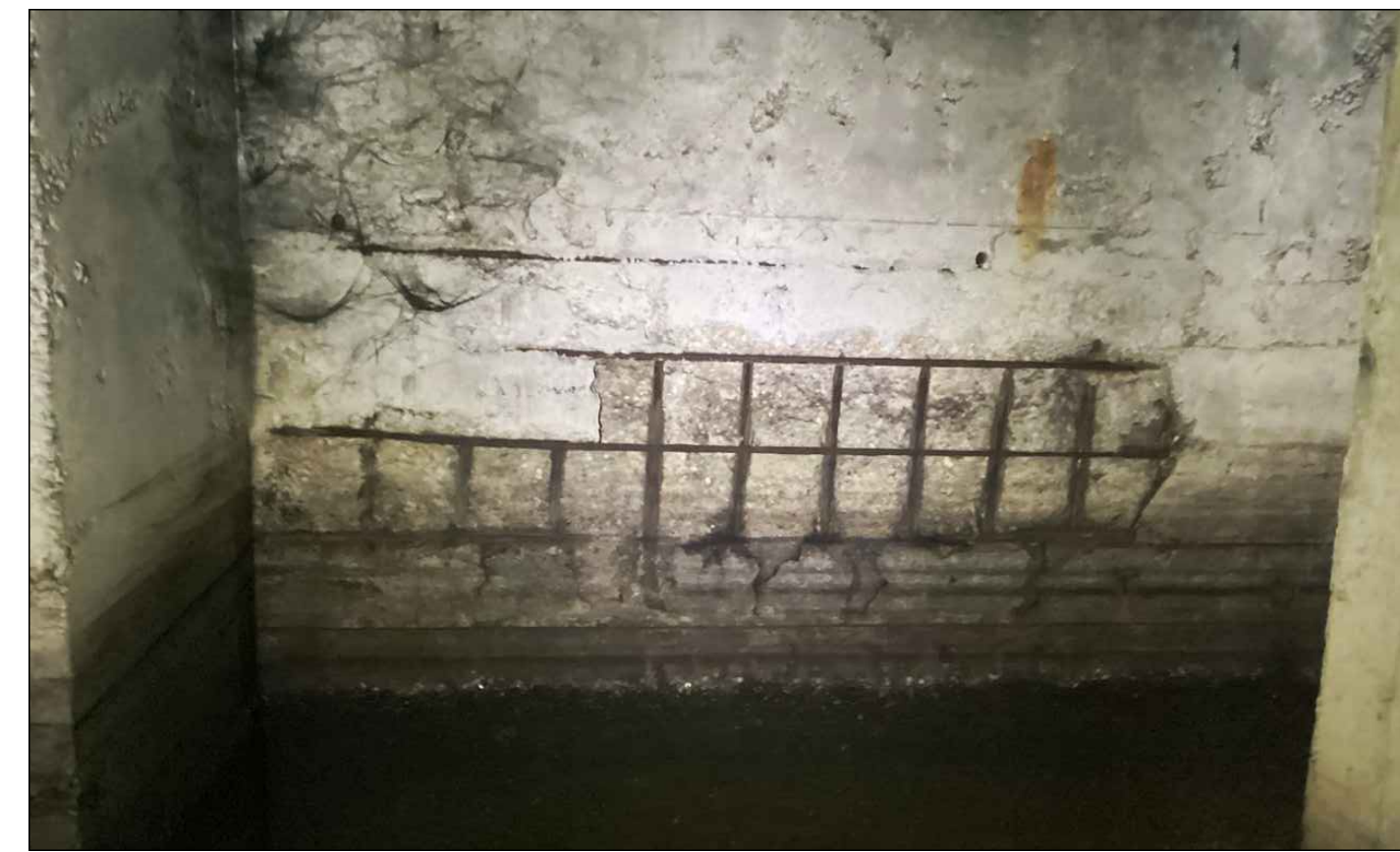
WALL DAMAGE REFERENCE PHOTO @ LOCATION 28 N.T.S.
