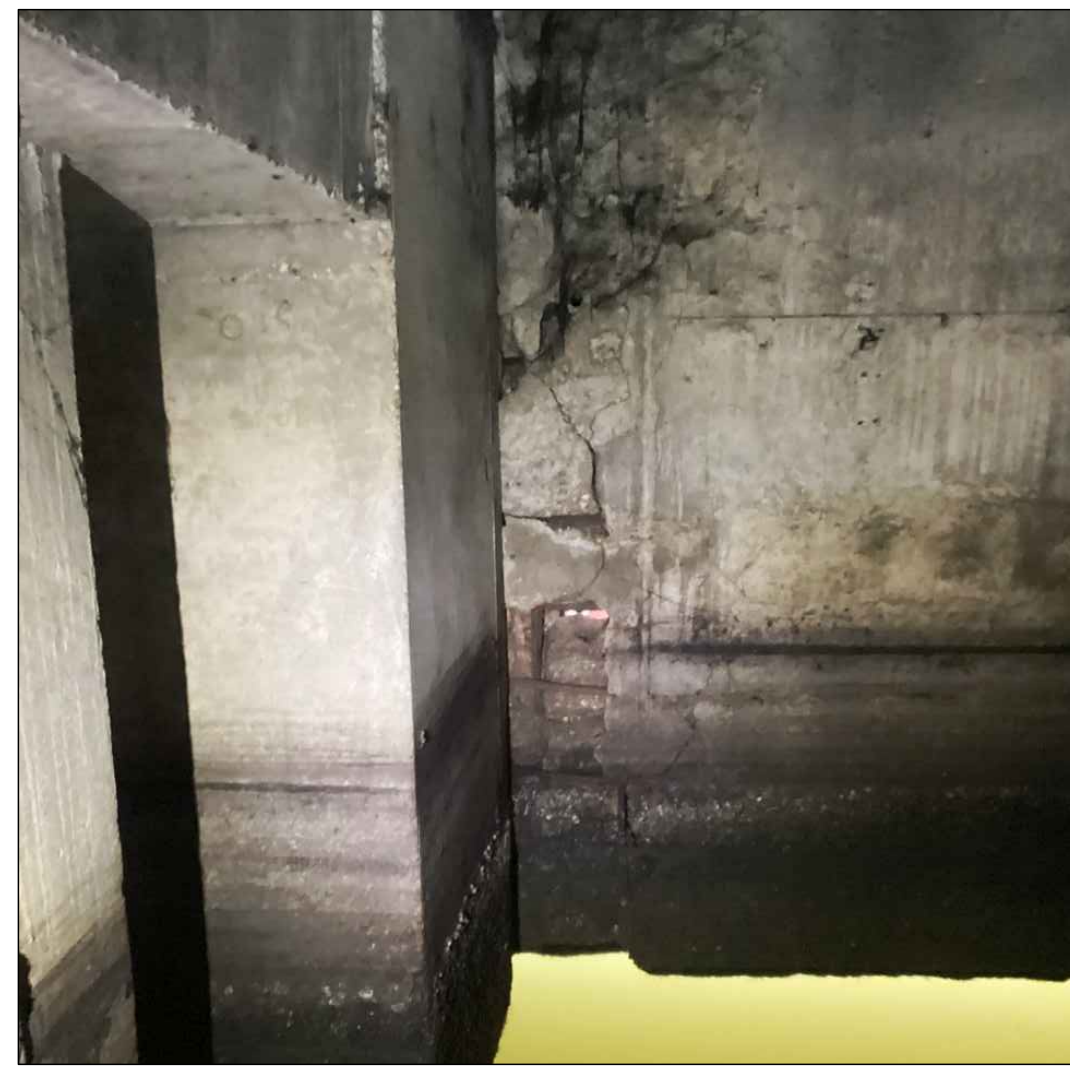
WALL DAMAGE REFERENCE PHOTO @ LOCATION 36 N.T.S.
